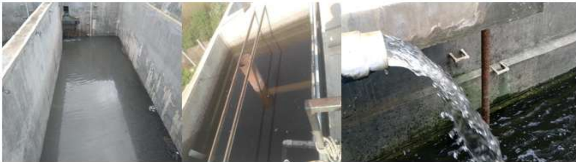
JMR Collection Tank, Settling Tank (after filtration)
