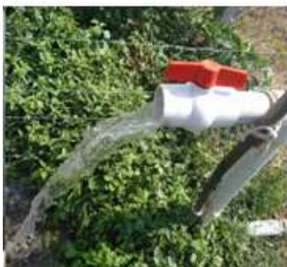
Outlet for the recycled wastewater from STP
