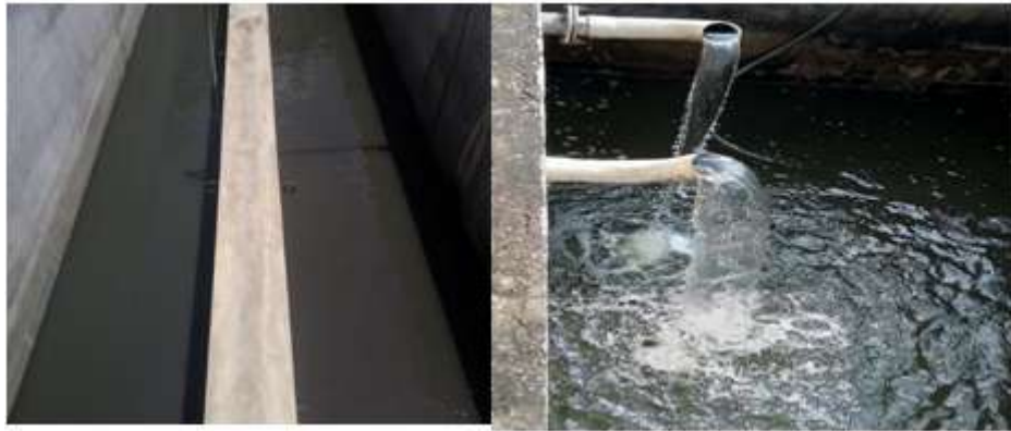
LH Collection Tank (After Filtration)
