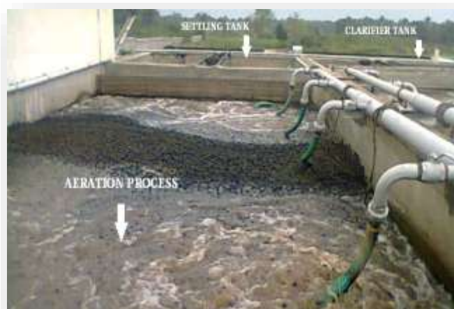
Fluidized Bed Reactors
