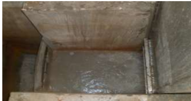
Sludge Drying Bed
