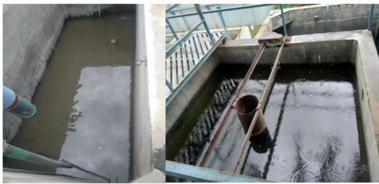
PRG Collection Tank, Settling Tank
