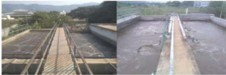
JMR and LH STP – Aeration Tanks
