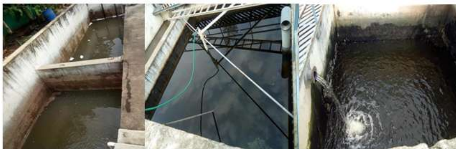
FDR Collection Tank, Settling Tank (after filtration)
